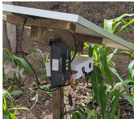
Plate 2: Solar Power Subsystem and Sensor Node Assembly
