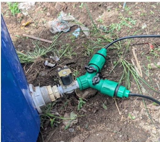
Plate 3: Overhead Tank with Irrigation Solenoid Valve
