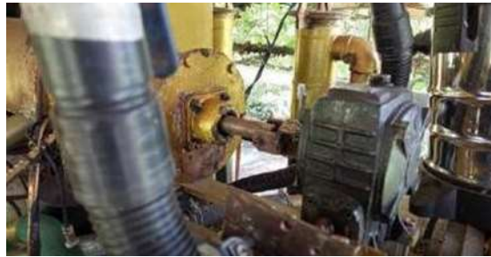
Figure 11.1. Functionality Test for the Motor (Auger Conveyor)
