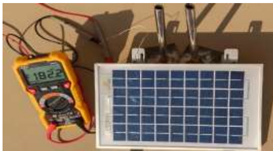
Figure 5. PV panel ampers
