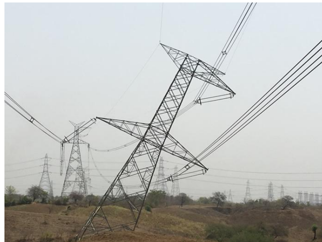
figure 2: Tower failure due to heavy wind load
