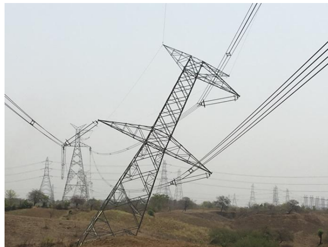
figure 2: Tower failure due to heavy wind load
