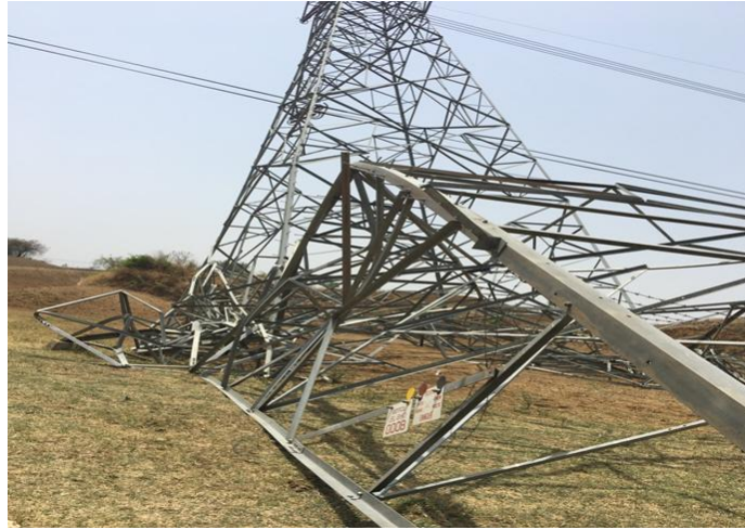
Figure 1: Tower failure incident near Bhopal (2019)
