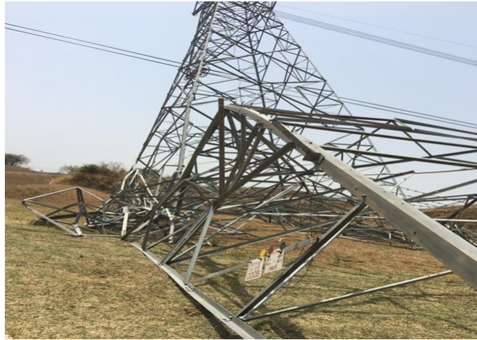
Figure 1: Tower failure incident near Bhopal (2019)
