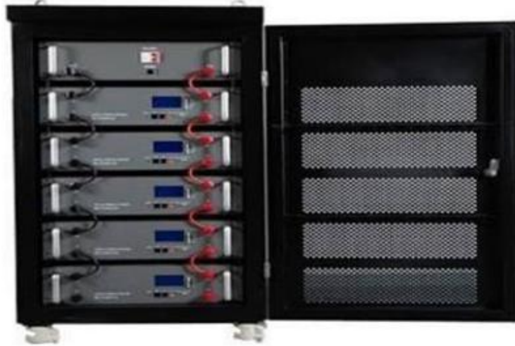
Fig 5: Battery storage unit
