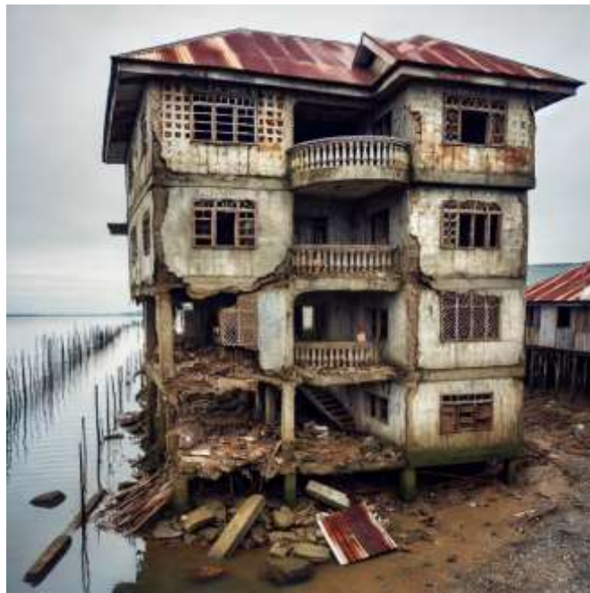
Plate 1: Exterior View of a Deteriorating Building in Bonny Island, Rivers State
