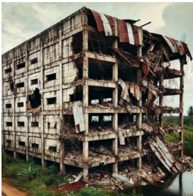
Plate 1: Coastal Building Deterioration in Forcados, Niger Delta, Nigeria
