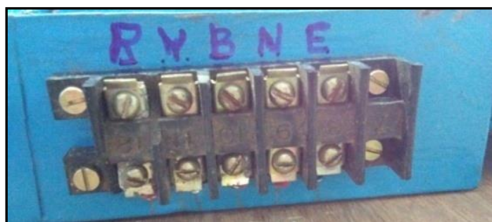
Fig (ii) Supply input terminal box
