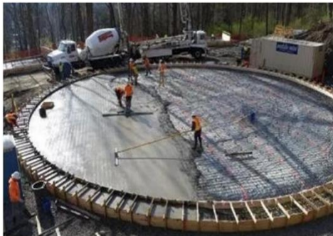
Figure 1.5 Reinforced concrete water tank floor above ground Floor of tanks rest on support
