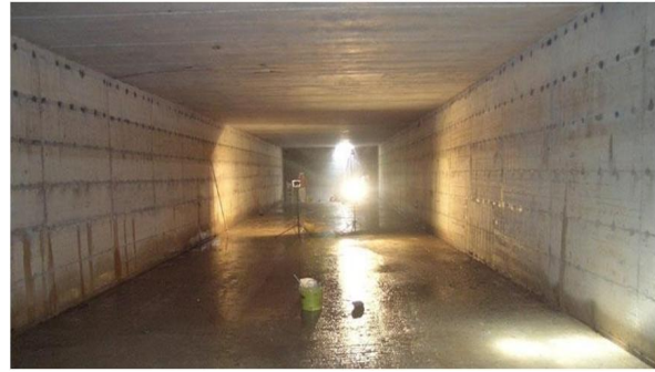
Figure 1.2 Underground Water Tank
