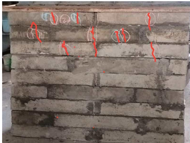
Fig.13 Crack after testing of conventional masonry wall
