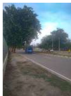
Figure 6. Surface Condition of the Pedestrian Pathway on Nicolau Lobato Street in Segment I
