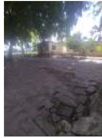
Figure 7. Surface Condition of the Pedestrian Pathway on Nicolau Lobato Street in Segment II
