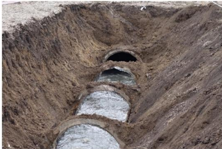
Fig. 1. Destroyed vaulted part of the reservoir.
