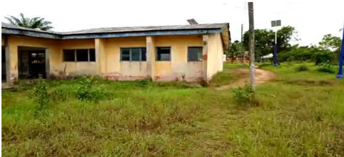
Plate 1: Dilapidated and Abandoned PHC Facility in Epellema Community in Opobo/Nkoro LGA
