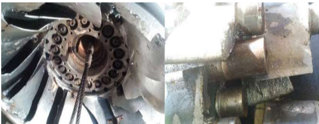
Figure 6-Erosion in 76 MW Francis turbine runner and guide vanes of MB-II Hydropower Plant
