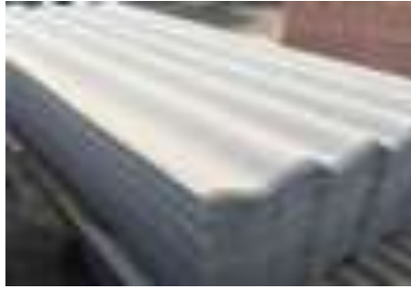
Fig 1: A Typical Example Of Asbestos Concrete
