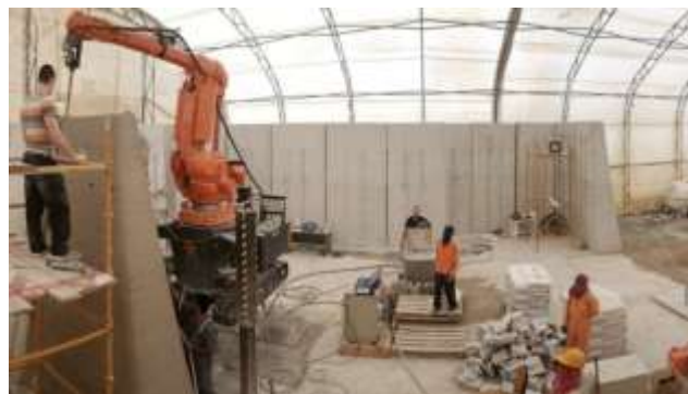
Fig. 1.7: The mobile construction robot CyBe RC 3Dp fabricating a drone laboratory by applying a concrete extrusion process on a job site in Dubai in 2017. (Bogue, 2018)
