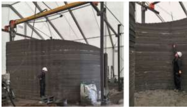
Fig. 1.3: Wall fabrication by utilizing a large-scale gantry system set up on the building. (Dörfler, 2018)
