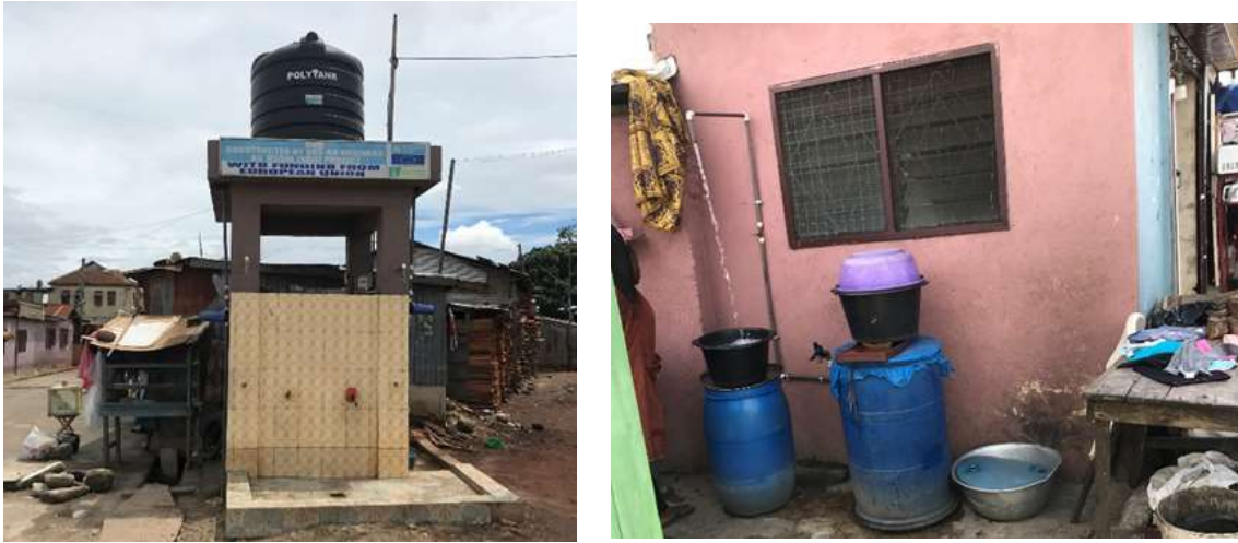
Figure 3.6.2: Mechanized borehole and standpipe (Source: Author's field study)
