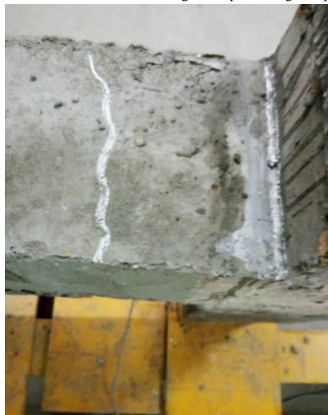
Figure 11: Crack formation of Precast connection
