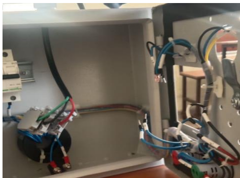
Figure 5 wiring completed in MCB
