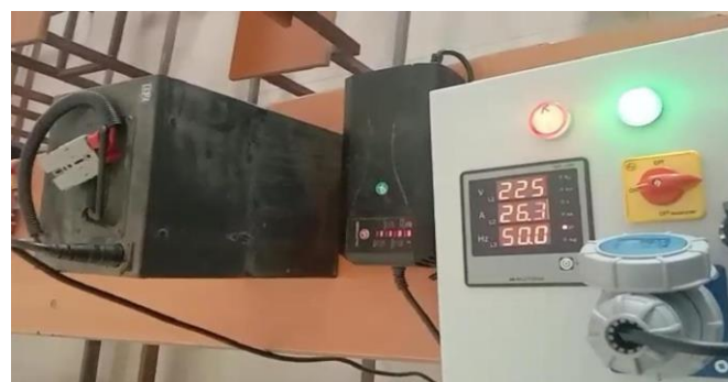
Figure 7 charging a battery
