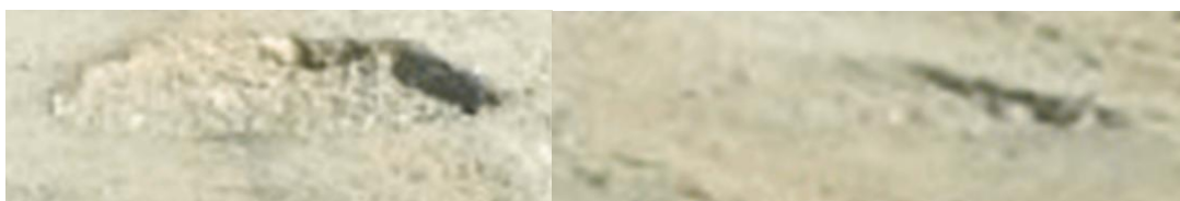
Figure 1. On the right, a sample picture showing a severe pothole and a moderate one on the left
