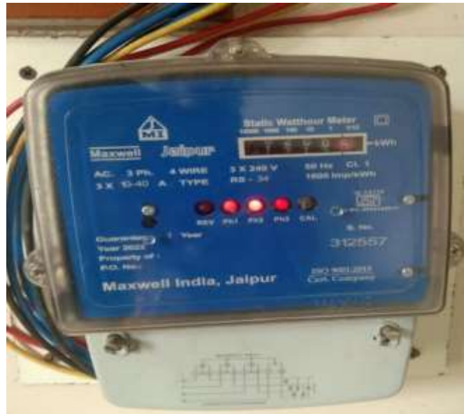
Fig I - Energy meter showing one month energy in kwh without our system/setup.
