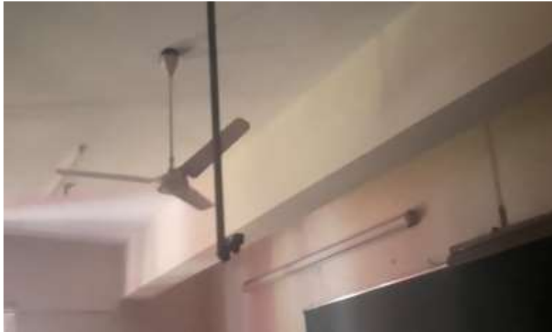
Fig F - All fans and tube lights of classroom are in OFF state room for checking
