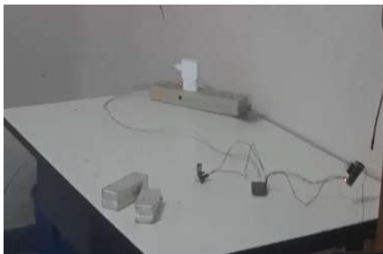
Fig E - Installed system in Classrooms
