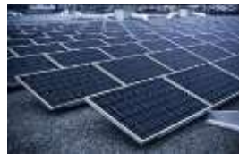
Fig:6 solar panels
