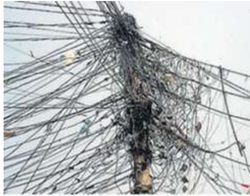
Fig.1. Power thefts from Electricity Poles
