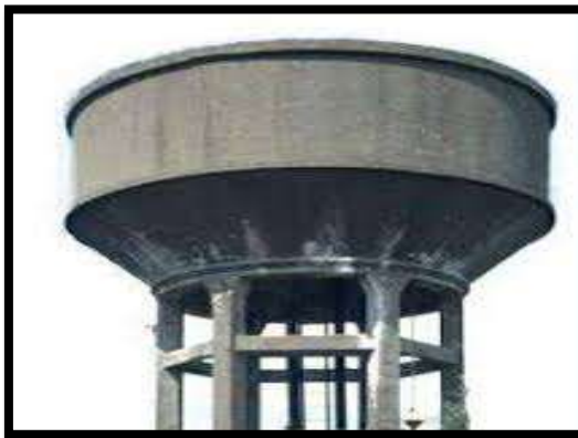
Fig no.3 Elevated water tanks Also, the water tanks are classified based on shape:
