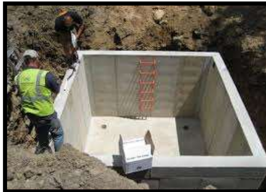
Fig no.2 Underground water tank
