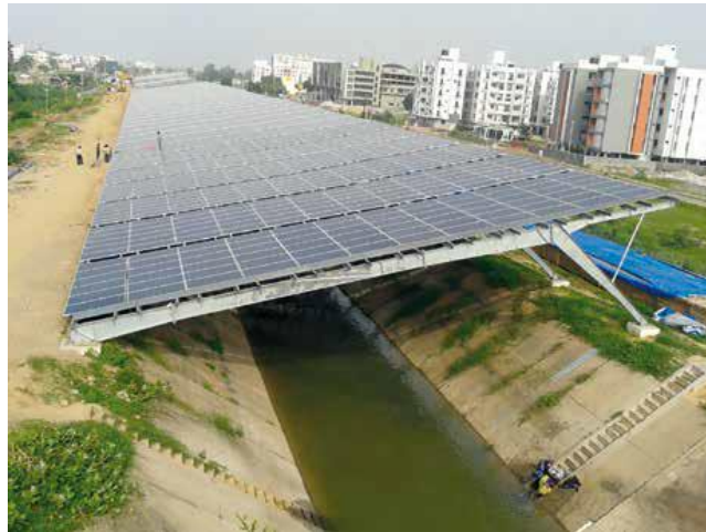
Figure 2: 10 MW canal top solar PV plant in Vadodara City, Gujarat
