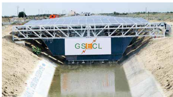
Figure 1: World's first demonstration of canal top solar PV plant at Chandrasan, Gujarat
