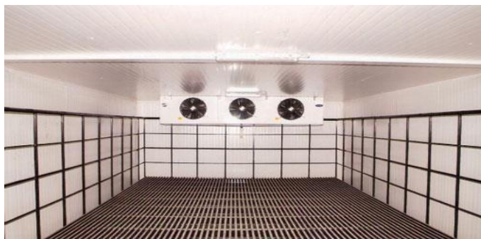
Fig.3.1 Evaporator located on the Top
