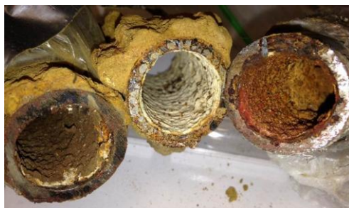
Fig. 2 - Rust and iron corrosion in flint drinking water pipes
