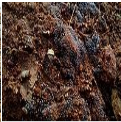
Mold on wet soil
