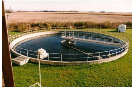
Figure - 11: Secondary settling tank
