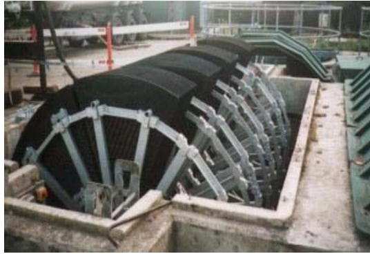
Figure -16: Rotating biological contactor
