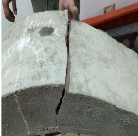
Fig 9: Major crack on arch
