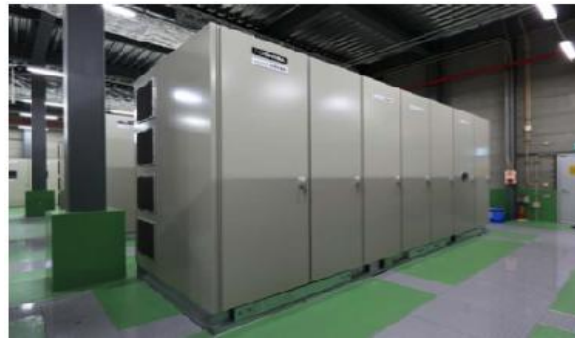
Fig 3 600 kVA power conditioning system (Noriko Kawakami, 2012)
